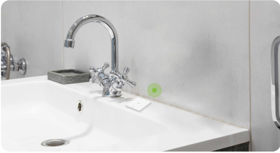
Bathroom (Toilet sinks, washing machine)
